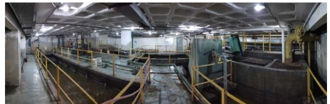
Fig. 2: The STP setup at the basement of the NSU
